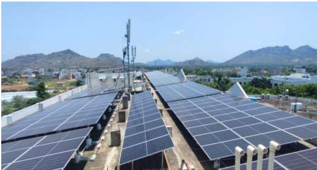
250 kW rooftop solar PV system on Saraswathi Block.
