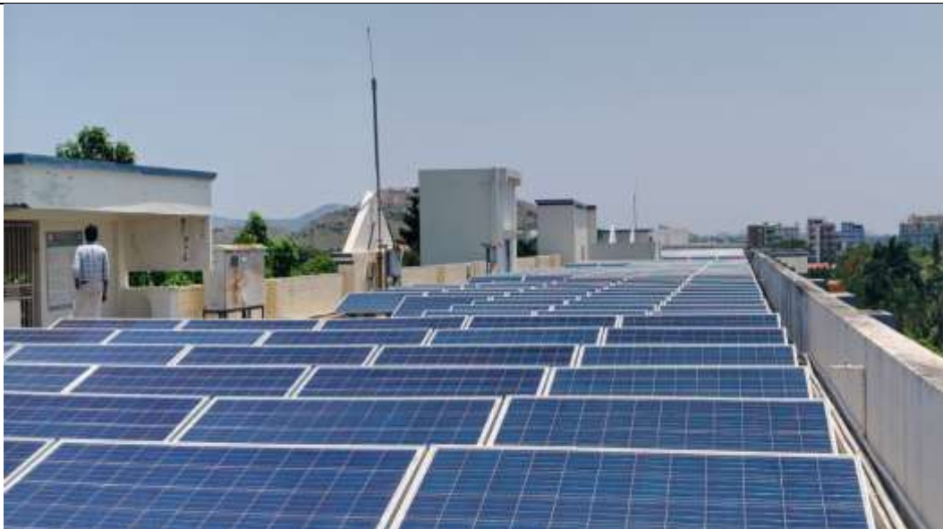
150 kW rooftop solar PV system on Lakshmi Block
