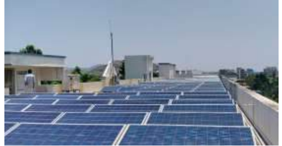
150 kW rooftop solar PV system on Lakshmi Block
